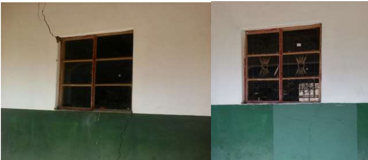
Figure 4: Structural crack at Sibusisiwe prior to repair after repair
