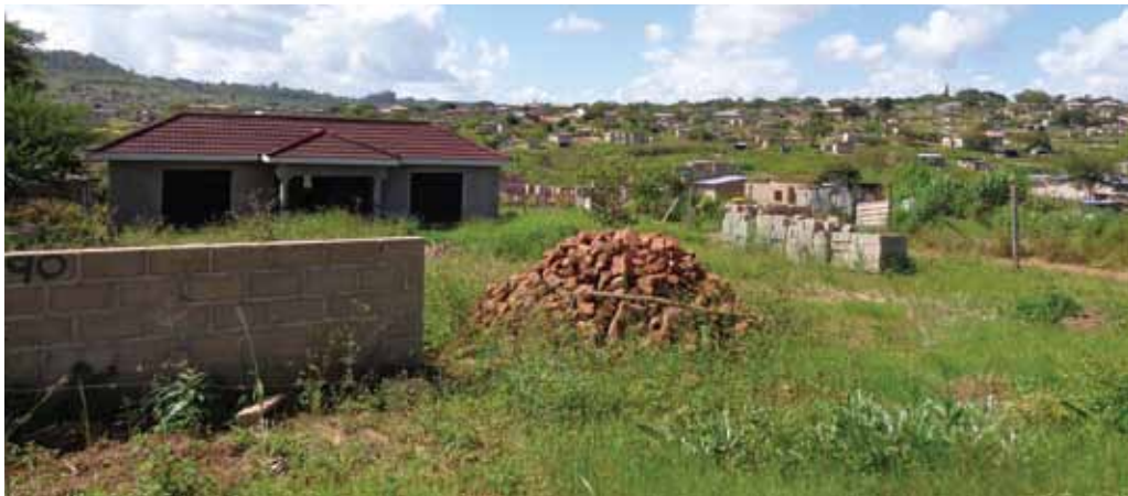
A house under construction. It is a good example of the size of many of the houses being built in the area.
