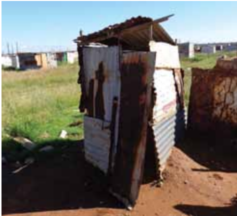
Pit latrines at Kamohela.
