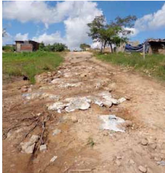
Uncontrolled runoff has eroded secondary roads in the settlement to the point where they are virtually impassable.
