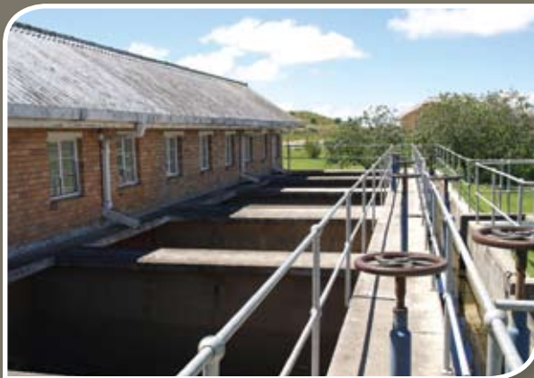
Waainek Water Treatment Works: Waainek Filters.
