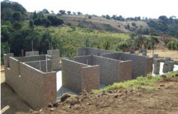
Rehoboth Foster Care Project: Construction of a new foster care home in Murchison situated in the Hibiscus Coast Municipality. PPT and the Ukulungisa Project Preparation Fund assisted the Rehoboth Trust in securing additional funding for the construction of 10 ten new homes. This project follows the success of the first phase in which 10 homes were built. Each home will accommodate 5 children and their foster parent.
