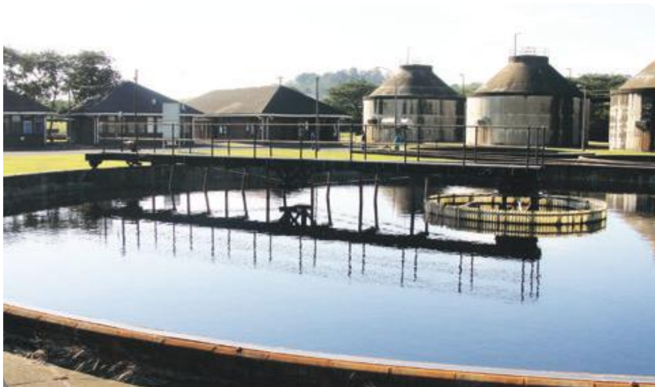
Sundumbili Waste Water Treatment Works Project: Through Ukulungisa, PPT successfully leveraged R12 million for interim upgrading and a further R219 million will be targeted for eventual full upgrading. Ukulungisa funded feasibility work and an application for capital funding from MIG.
